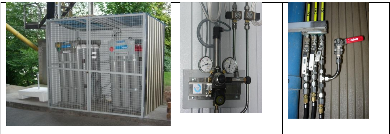
Fig. 5: Components of gas supply: gas cylinder bundles; pressure reduction station; ball valves at each generator
