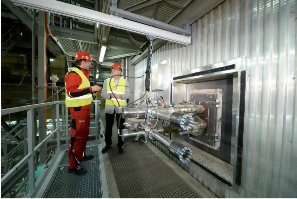
Figure 2: Installed TwinL Shock Pulse Generator in Waste to Energy Plant Zurich Josefstrasse
